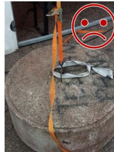
Figure 12. The S hook will come loose as wind moves the structure. The fastening is not locked to the mounting point.
